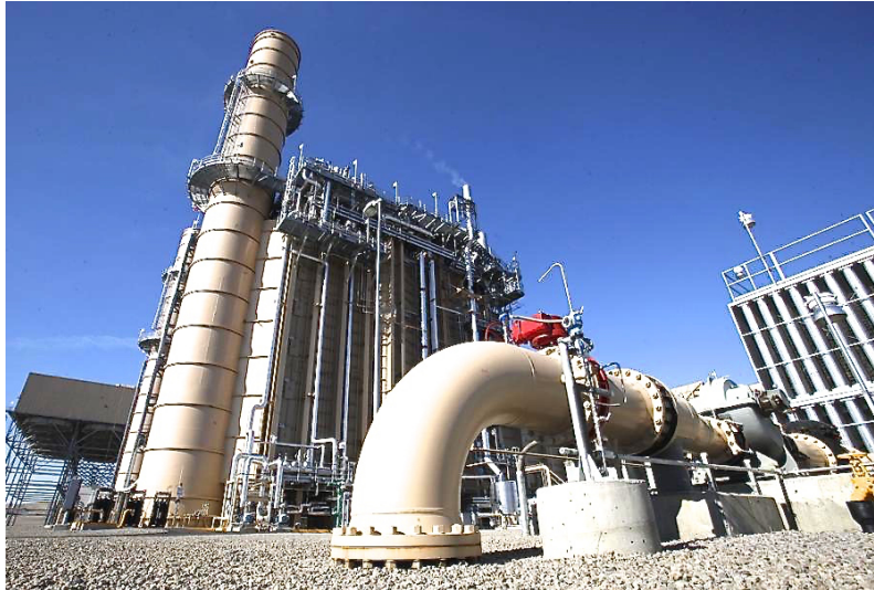
Pacific Gas & Electric's Colusa Generating Station has operated at well below its generating capacity — just 47% in its first five years. (Rich Pedroncelli / AP)
