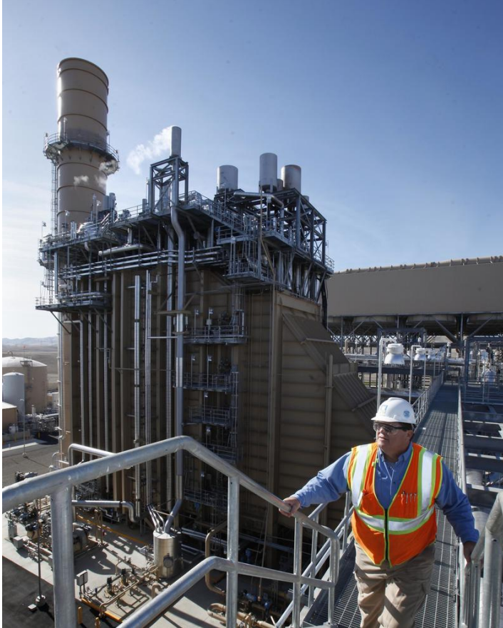
Colusa Generating Station opened in 2010. Pacific Gas & Electric will charge ratepayers more than $700 million over the plant's lifespan, to cover its operating costs and the profit guaranteed to public utility companies. (Rich Pedroncelli / AP)
